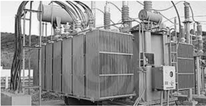
Figure 10: Electric power step-down station Source: Google.com
